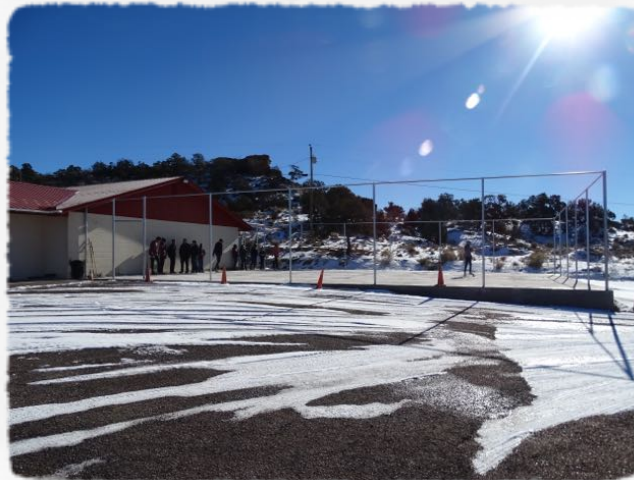
You can see the snow on the driveway. Concrete was finished before the snow came although we did have to cover it with concrete blankets many nights because of temperatures dipping into single digits.
