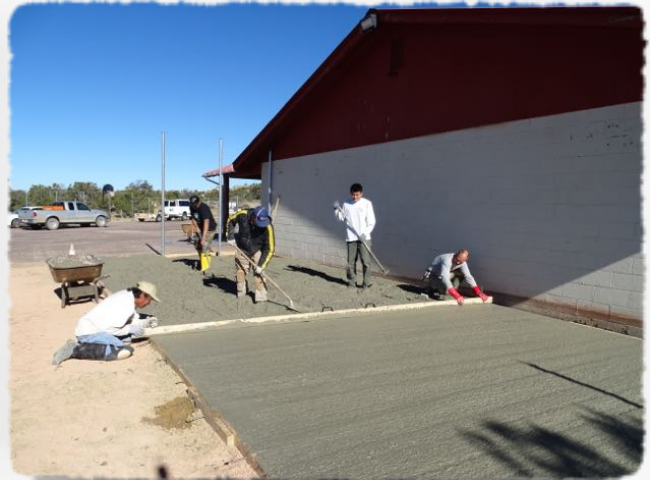
The first pad of concrete is poured and worked. This is the first of four pours.
