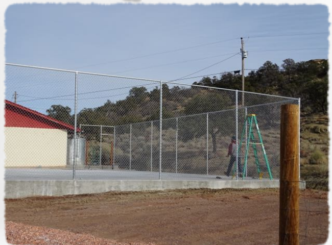
Fence is up, but gates still need to be installed which Jim will do himself.
