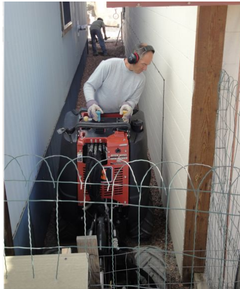
Jim and Les work on cutting a trench between buildings for the water line
